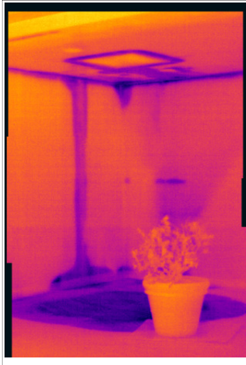
Figure 21. Fire sprinkler system leak observed on an interior painted wall and carpet. Initial wetting and drying appear much defined.
