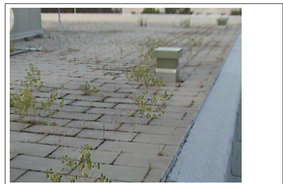
Figure 2. Visual of concrete clad insulation over inverted roof membrane, no visible wetting on concrete.
