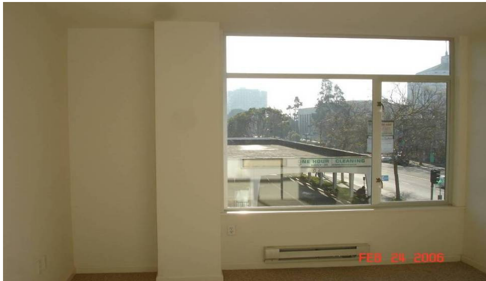
Figure 25. Interior surfaces of exterior walls showing no visible wetting other than flooring.
