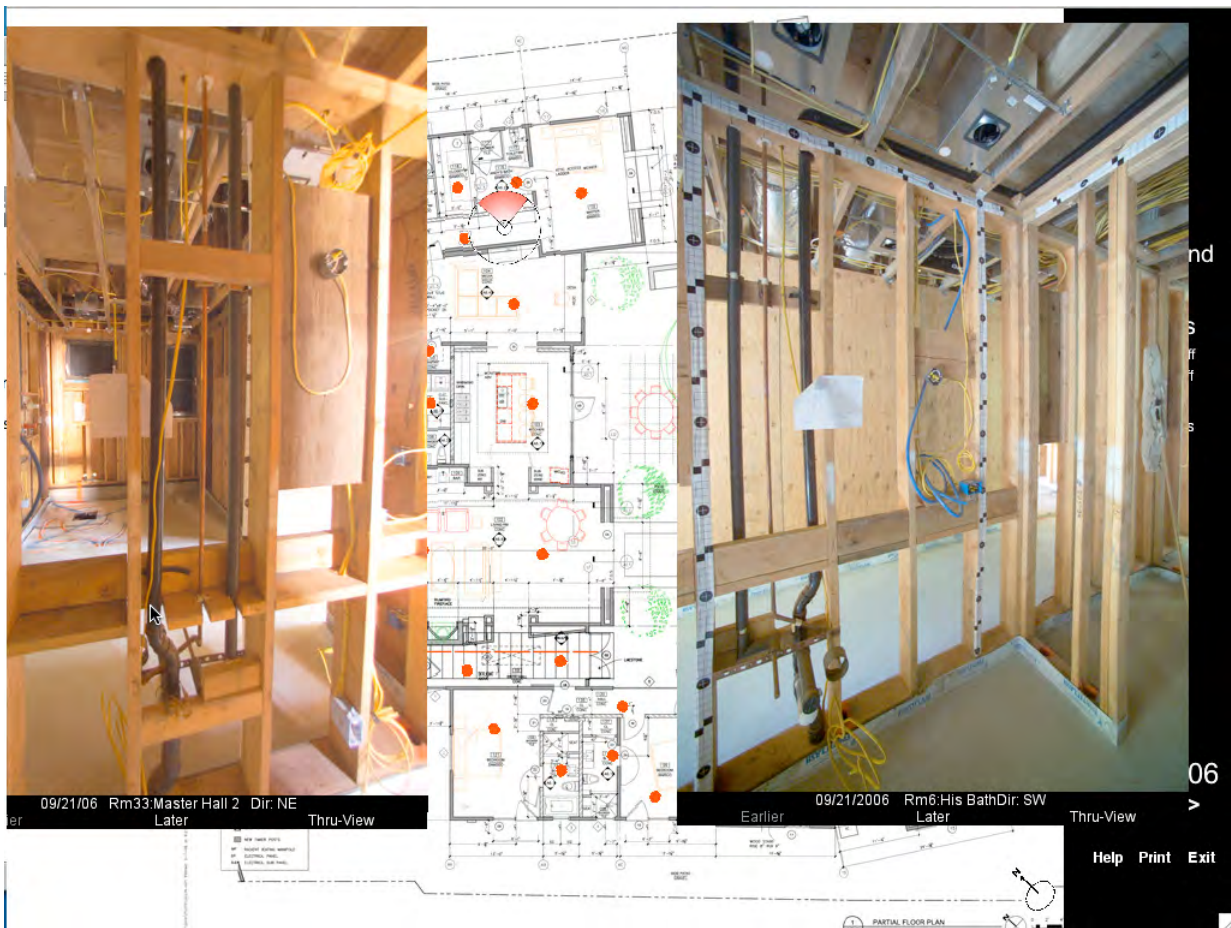
Figure 1. Screen shot of Imaging Perspective's viewer showing piping in bathroom from both sides of wall.
