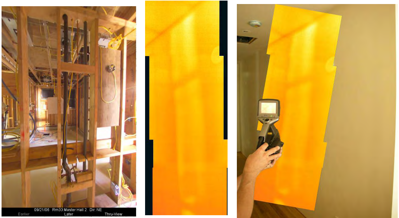
Figure 3. Visual and thermal images of vent pipe (leftmost pipe in stud bay) and hot-water pipe (rightmost pipe)
