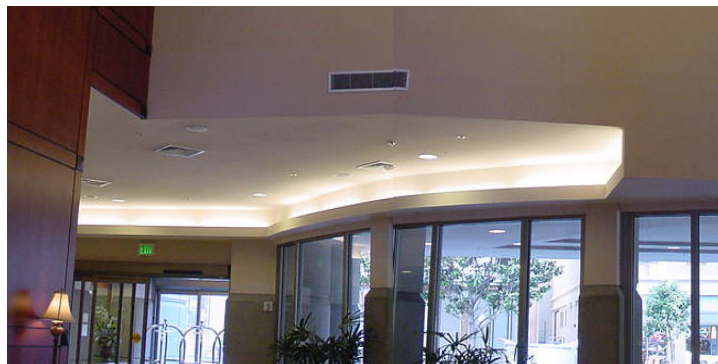
Figure 2. Thermogram/photo pair showing moisture detected on the ceiling of a hotel lobby.
